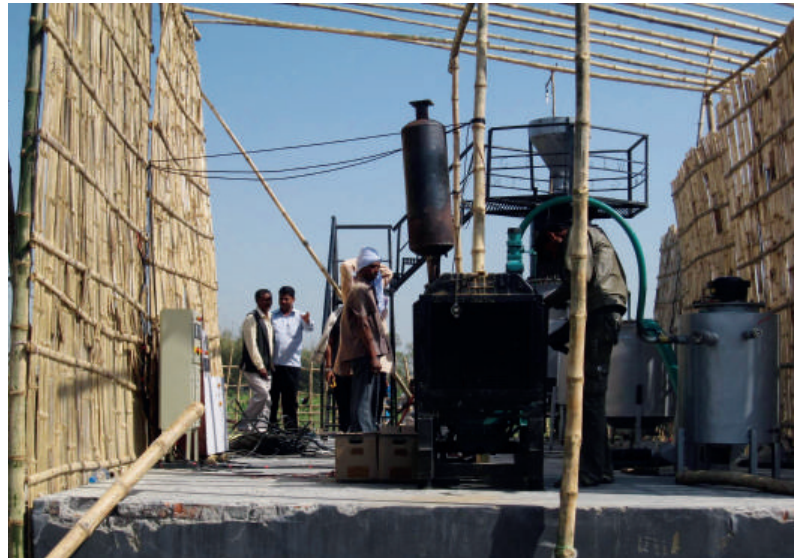
Power house Electricity is generated from rice husks in Bihar
